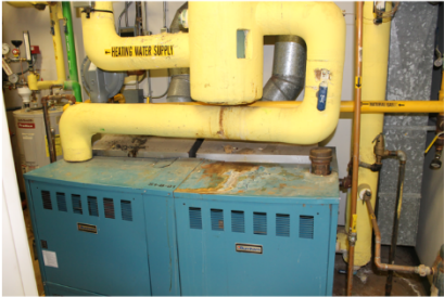
HOT WATER BOILER
